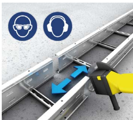
31 | Cutting Cutting must be performed with the greatest care, complying to all industrial safety regulations.
